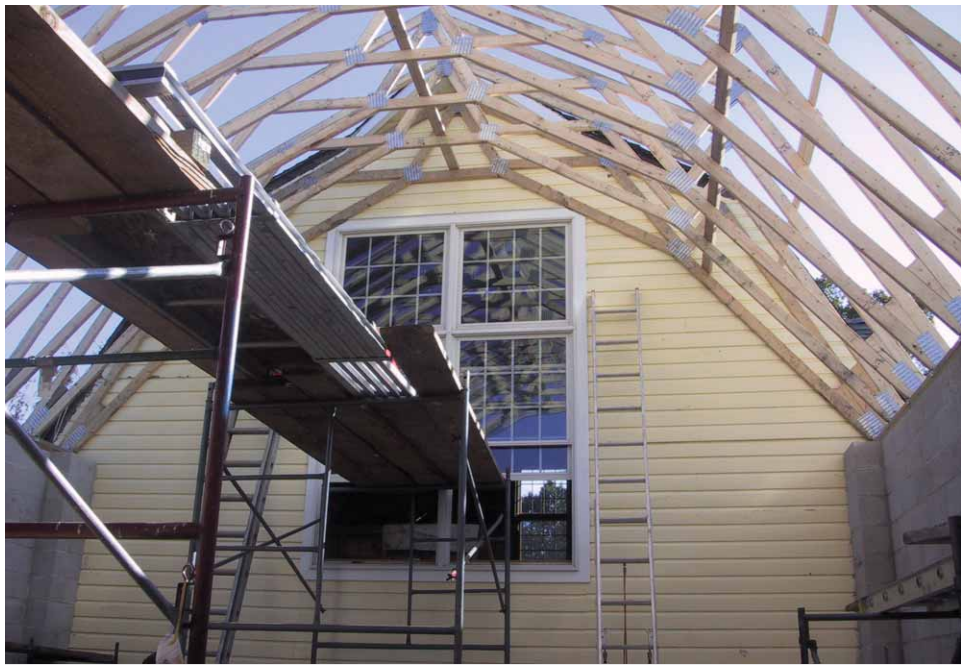
When planning their new barrel room, Crossing Vineyards’ owners referred to their business plan and built for the future.
